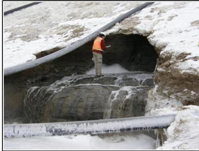
Figure 3-1 Piping Failure in Tailings Embankment
