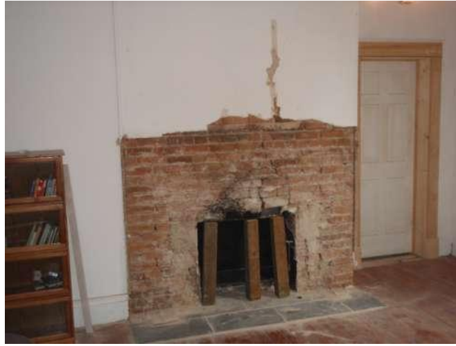
Figure 6-2 Damage Resulting from August 23, 2011 Earthquake
