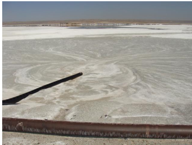
Figure 3-4 Tailings Discharge Piping
